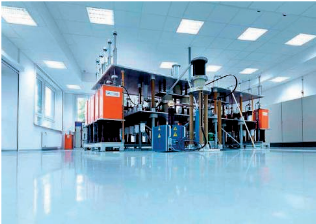
Lightning current generator
